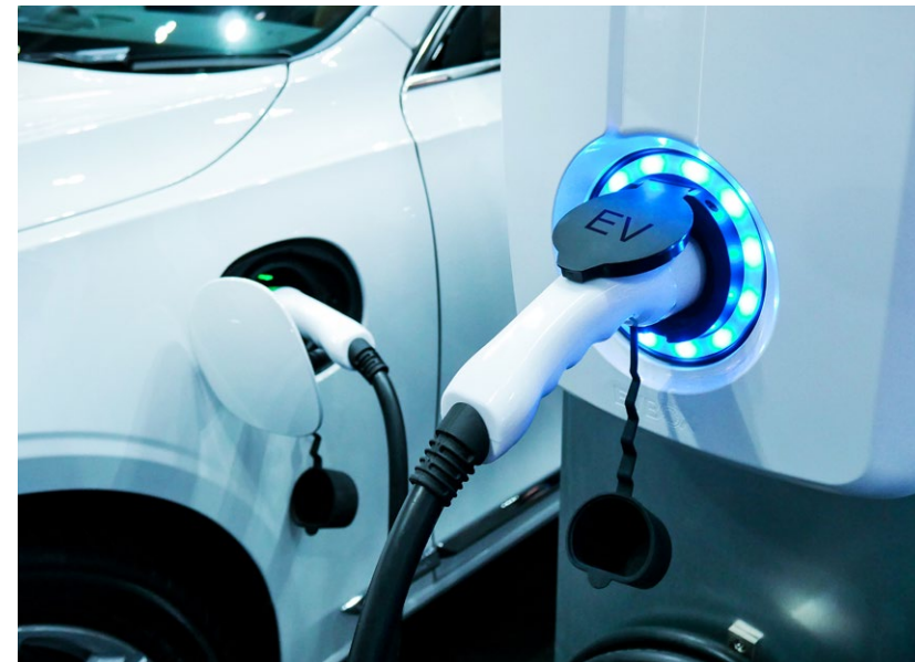
EV Charging Point
