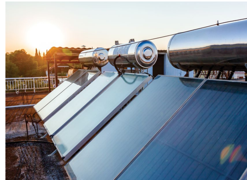
Solar Water Panels on Rooftop
